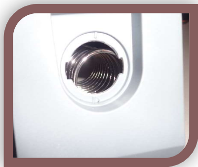
Misaligned (Off center).
